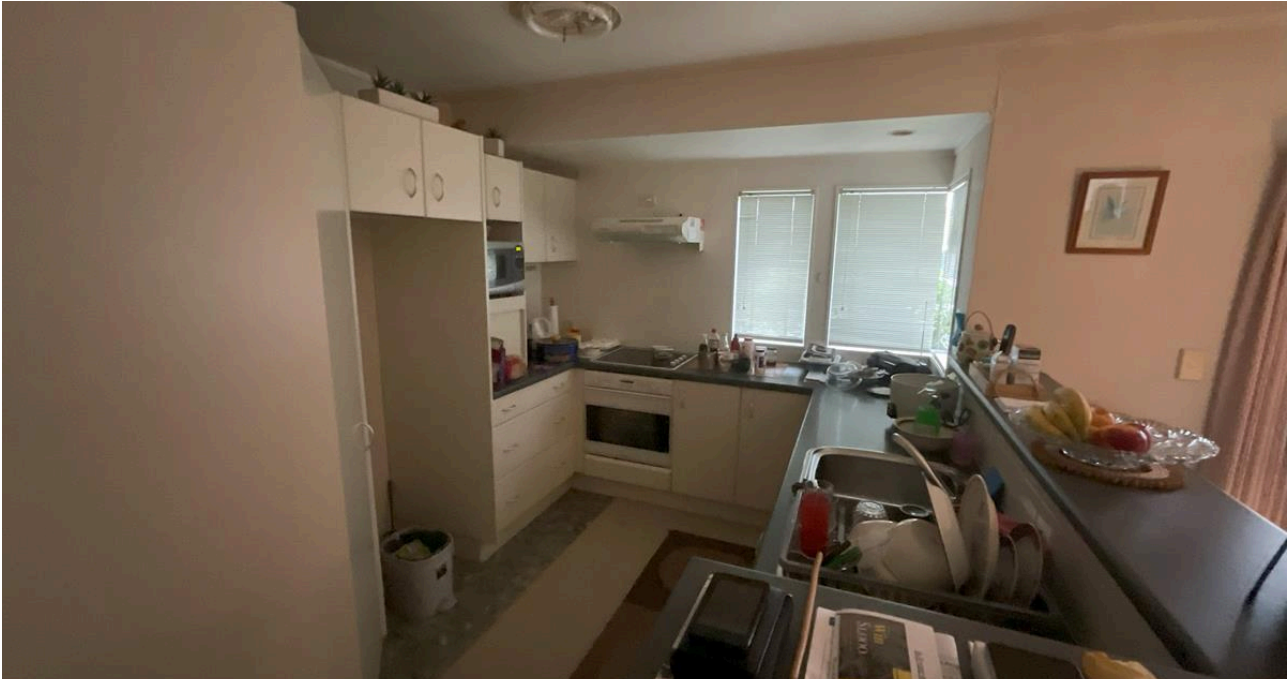
The original kitchen — a closed U-shape, walled off from the dining and living.
